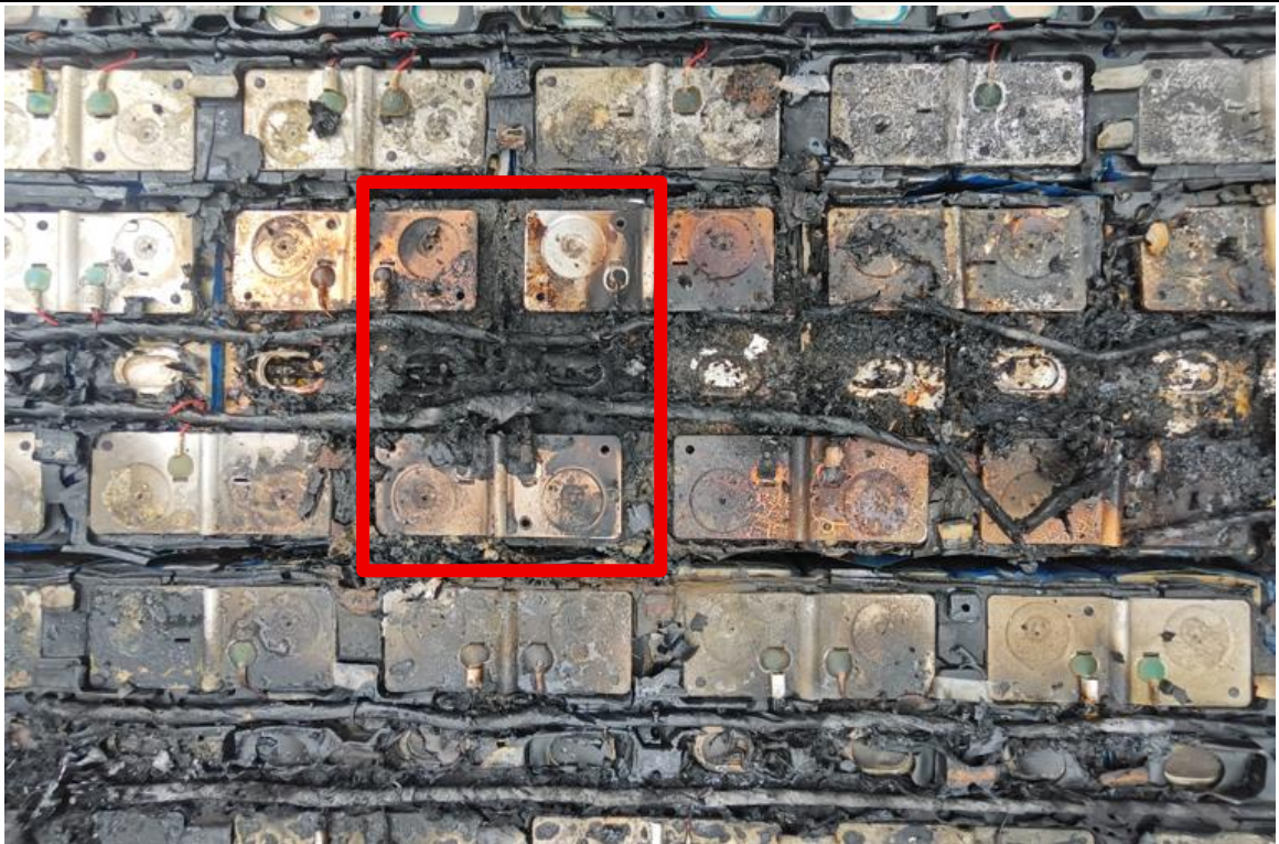
3 cells relief valves ruptured (cell 31 to cell 33) 2 cells thermal runaway induced (cell 32 and cell 33)
