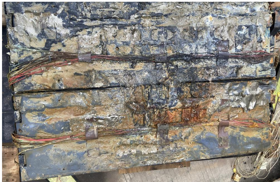
Figure 5 of Attachment 5 Internal of initiating module_after test
