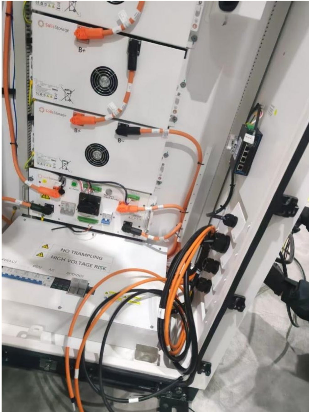
Figure 6- 1 Pre-installed cables inside cabinet
