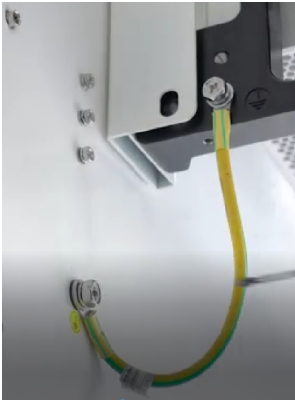
Figure 7-6 Ground connection with cabinet enclosure
