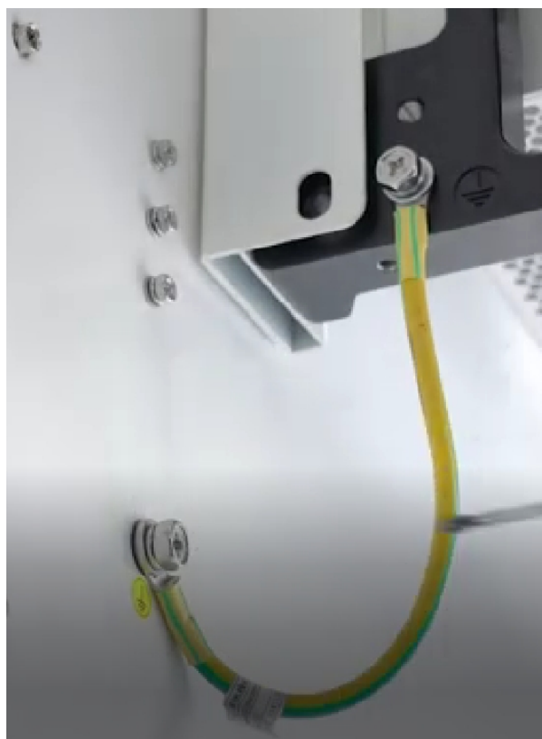
Figure 4-6 Ground connection with cabinet enclosure
