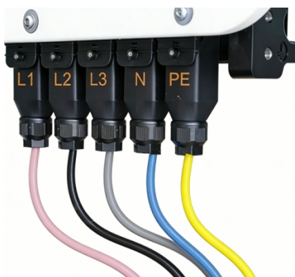
Figure 4- 19 Backup port auxiliary cable connection
