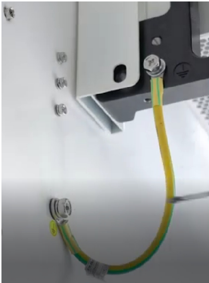
Figure 7-6 Ground connection with cabinet enclosure
