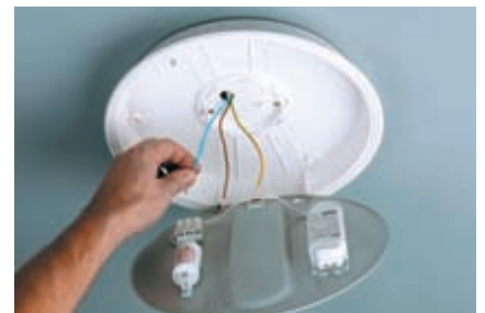
The wires are connected to the spring terminals
