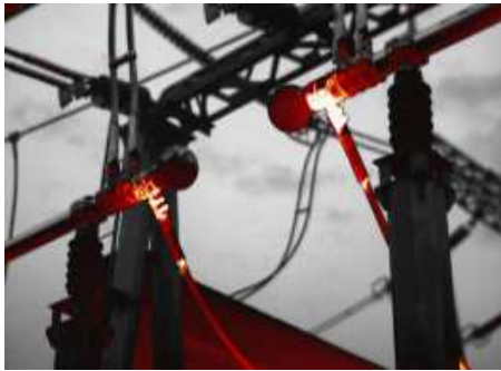
Clips Scan the whole line, to find hot spot. Usually failures happens on the bus clips.
