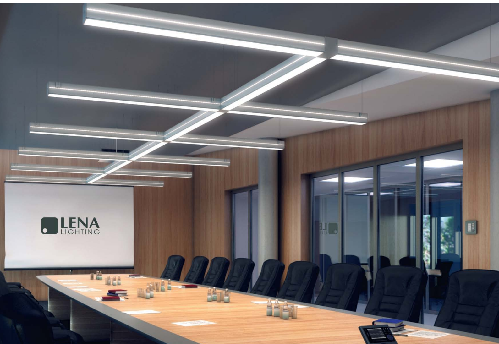
APPLICATION OF INTEGRA LED SYSTEM FOR BOARDROOM ILLUMINATION.
