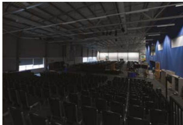
Space layout 1 – during LMS programming, it was possible to control each luminaire individually and not only according to the preset groups
